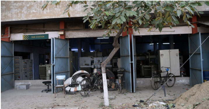
View of the Substation building taken in October with partially installed panels.
